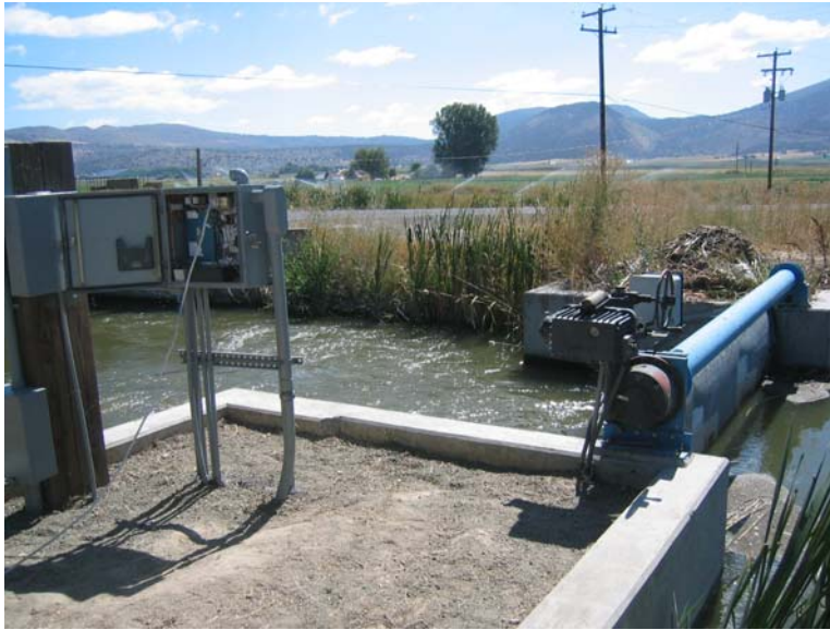
Figure 3. Automated flow rate control on the B Canal radial headgate.
