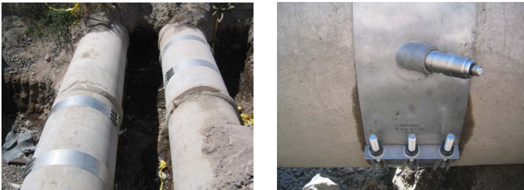
Figure 6. Existing concrete and steel pipelines at Miller Hill Pumping Plant showing the saddles used to install GE Panametrics wetted transducers.
