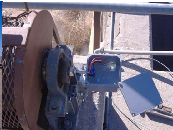
Figure 6. Gate Shaft Monitor
