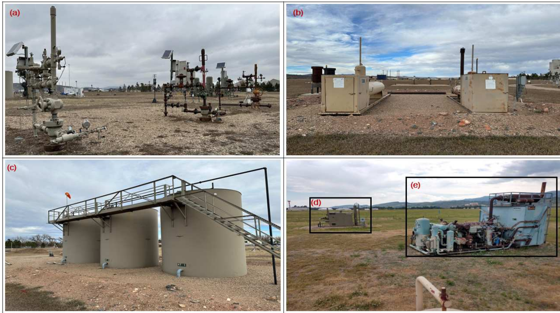
Figure 2.2: Figures (a), (b), (c), (d), and (e) show examples of decommissioned wellheads, separators, condensate tanks, a dehydrator, and a compression station available at METEC. The equipment units were donated by METEC’s Industry Advisory Board (IAB) during the construction of the facility in 2016.
