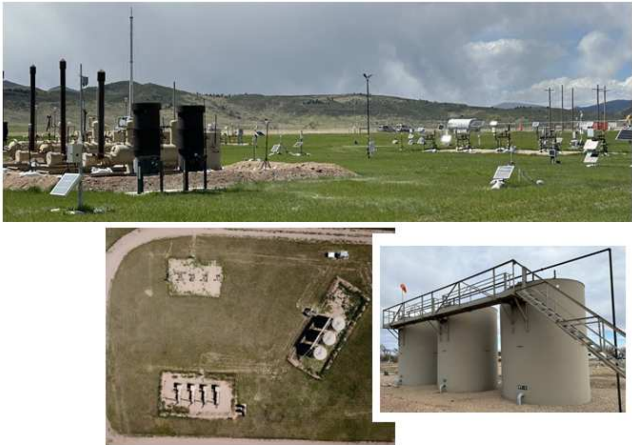
Figure 2.5: Well pad 4 is a 60 m × 60 m wet gas production facility consisting of 5 wellheads, 4 horizontal separators, and 3 liquid storage tanks.
