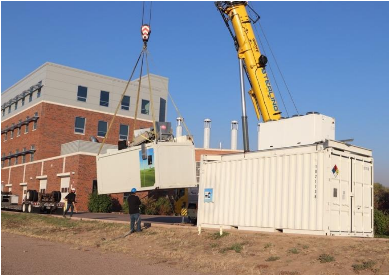
Figure 30: Nel Hydrogen vehicle refueling station being installed at the Colorado State University Powerhouse Campus [37].
