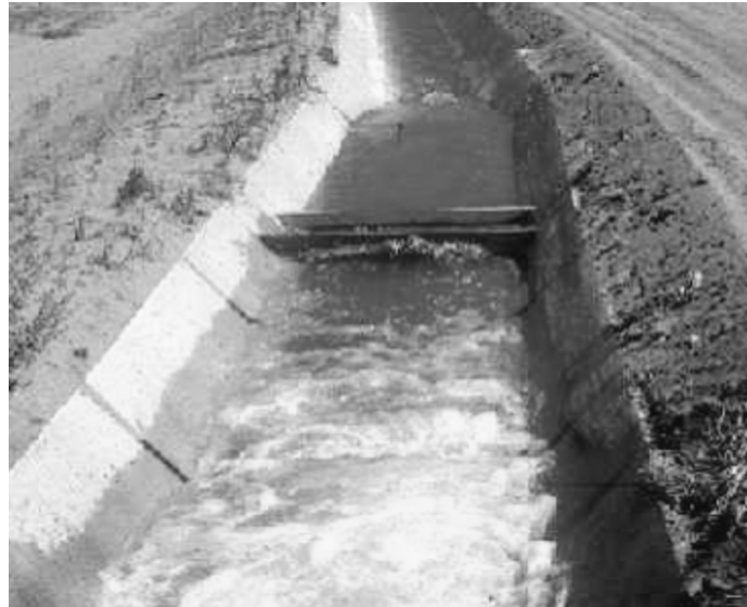
Figure 6. Wave Suppression in Small Canal.
