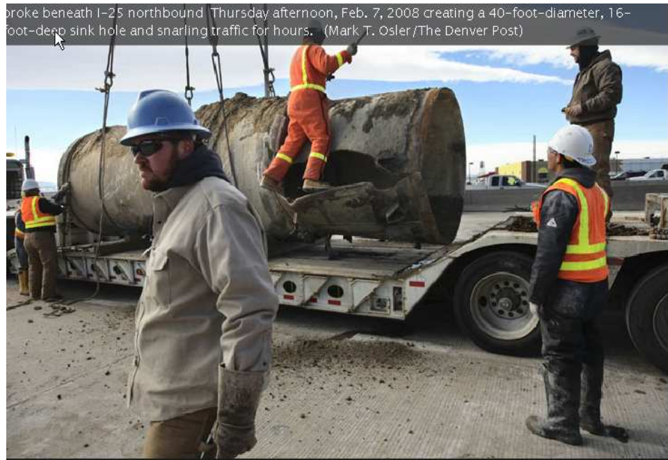
Figure 3. 66-in water main ruptures, I-25 in Denver (Leslie, 2008).
