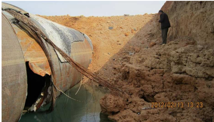
Figure 16. Pipe burst at station 76+860 in the Ajdabiya-Sirte pipeline system (personal communication, August 28, 2012).
