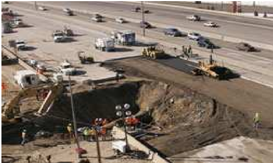
Figure 2. 66-in water main ruptures as a result of hydraulic initiated by a pump failure beneath the I-25 in Denver (Leslie, 2008).
