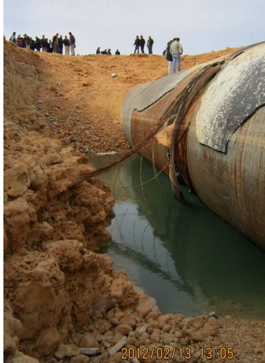
Figure 4. 4-meter diameter pipe burst in Libya in February 2012 (personal communication, August 28, 2012).
