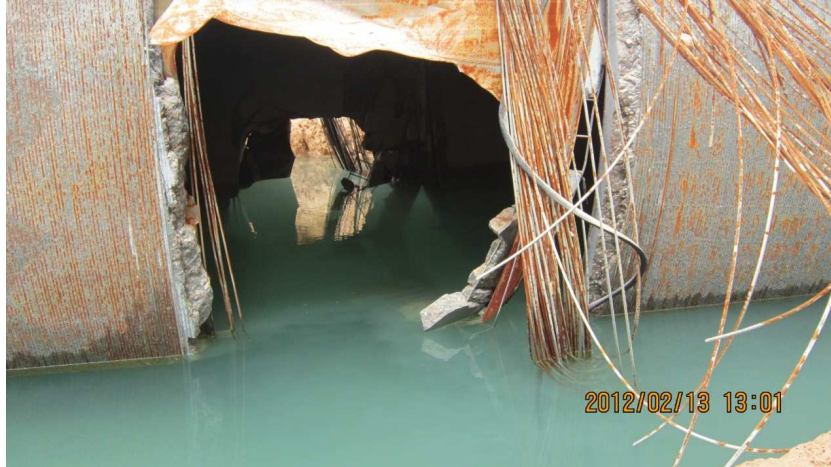
Figure 17. Pipe burst at station 76+860 in the Ajdabiya-Sirte pipeline system (personal communication, August 28, 2012).
