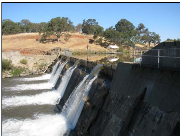
Figure 2. 2008 Pilot Water Transfer Weir Configuration.
