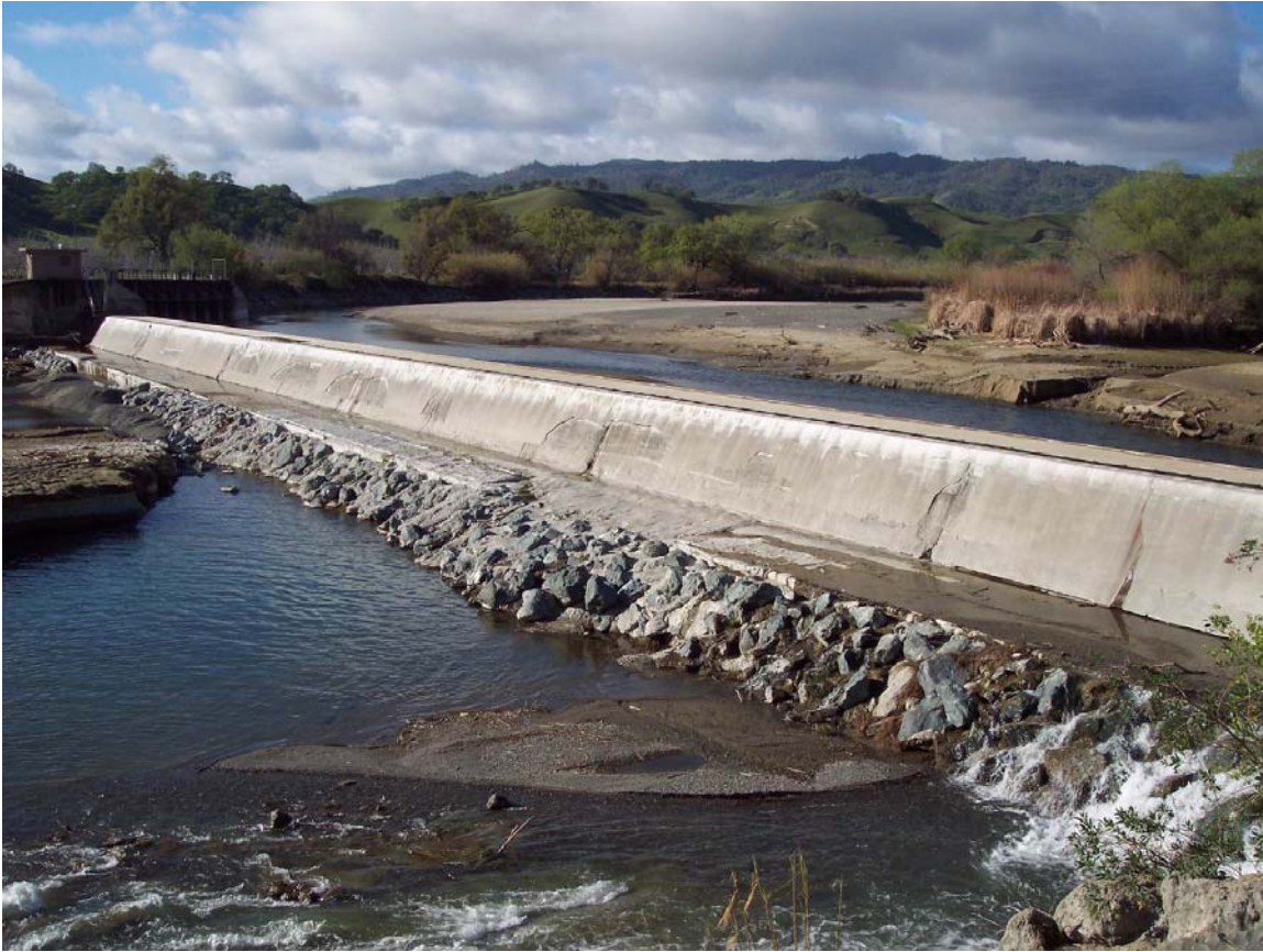
Figure 3. Photo of Capay Diversion Dam showing Cache Creek streambed degradation and local scour at end of apron
