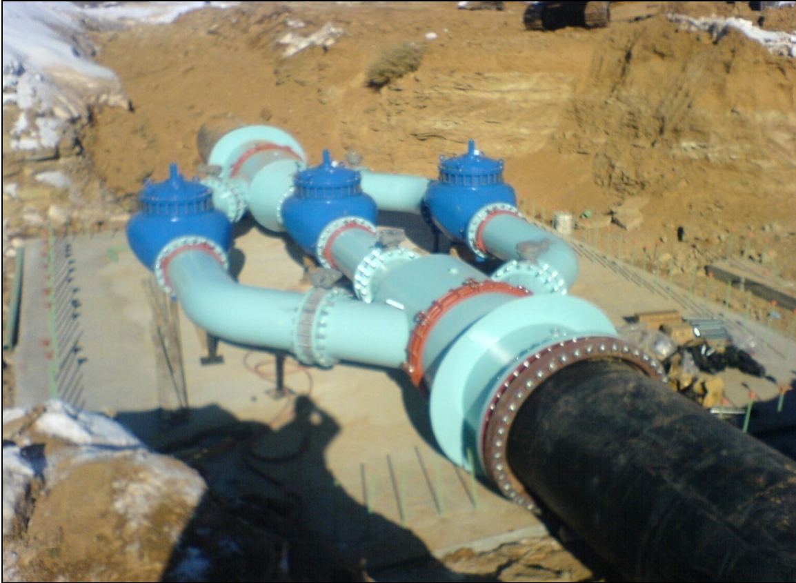
Figure 2. Pressure Reducing Valve Vault
