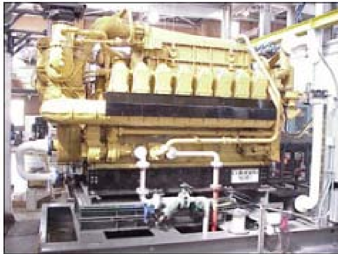
Figure 30. Caterpillar G3516C engine at the CSU-EECL.
