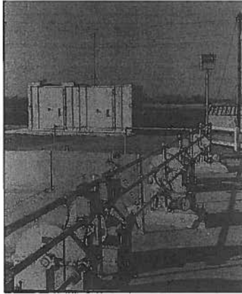
Fig. 6 Prefabricated control building
