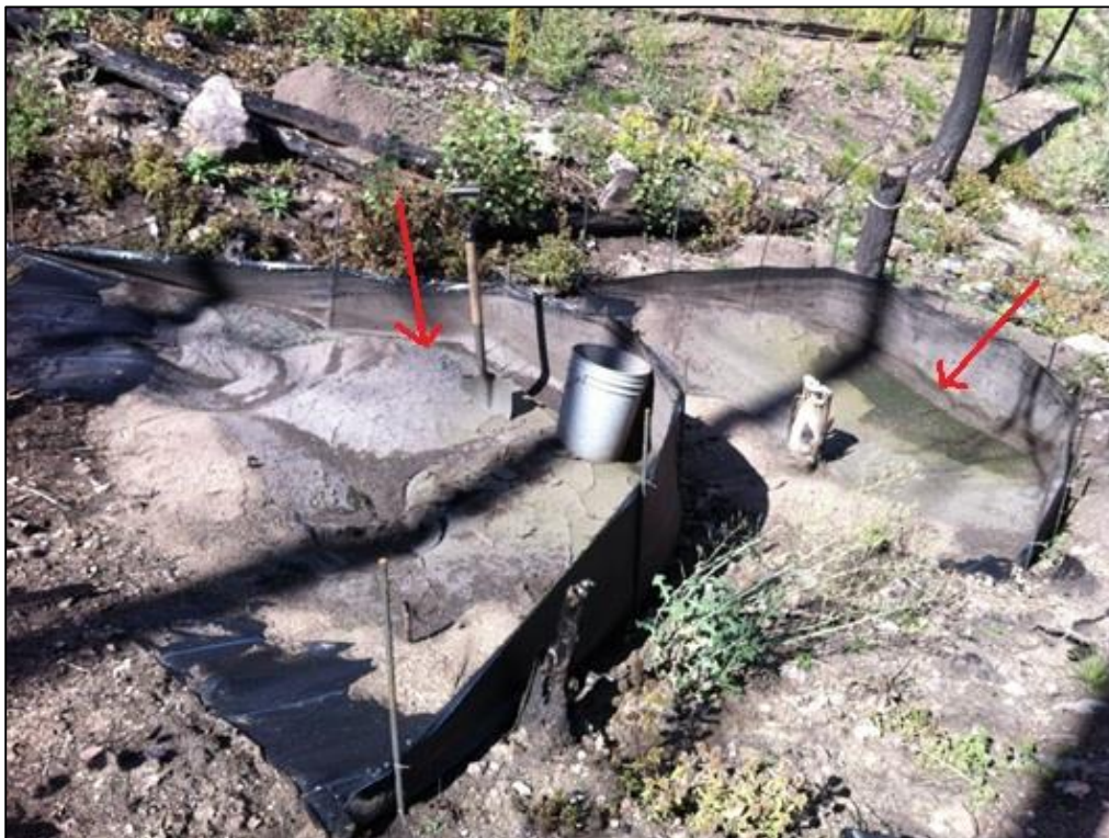
Figure 3.4: Photo of the double sediment fence at swale SM2 showing the amount of sediment in the lower fence that was not trapped by the upper fence. Red arrows point at the level of sediment in each fence.
