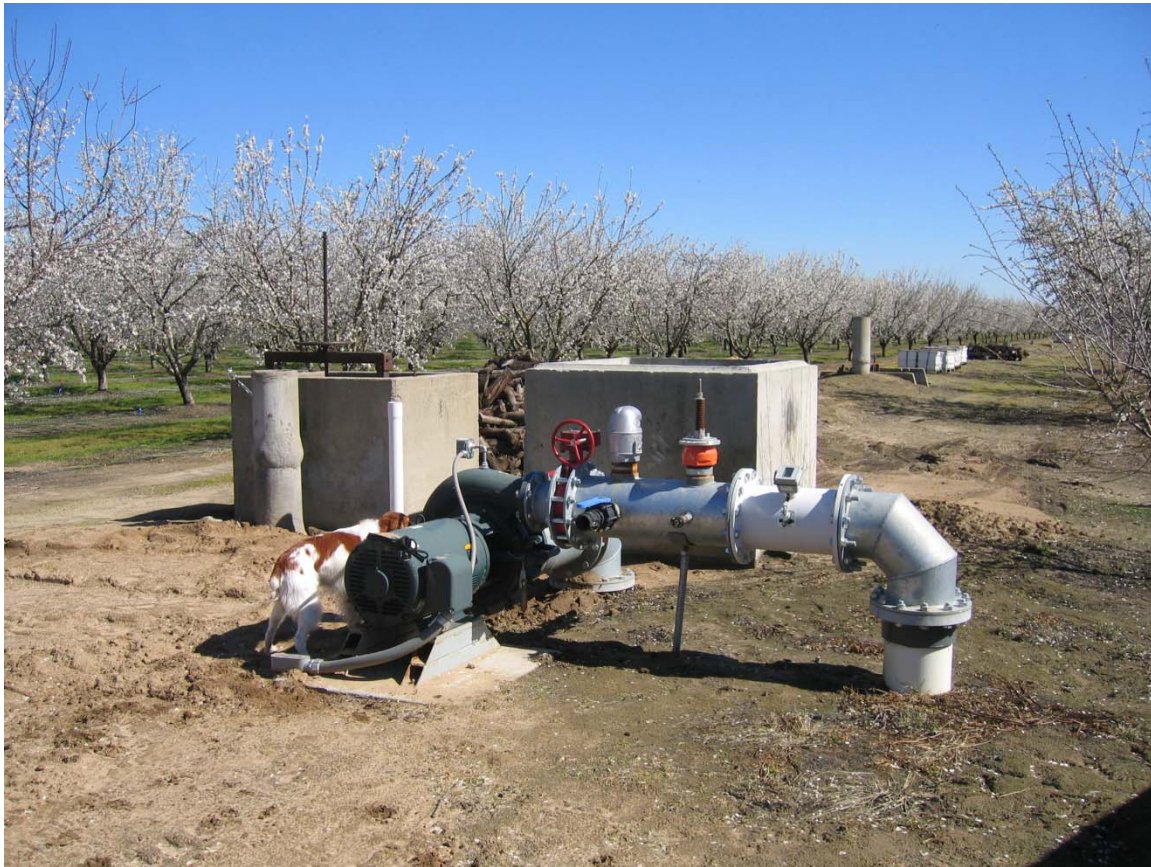
New Pump and Turnout/Moss Screen Box
